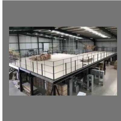
Mezzanine Storage Rack
